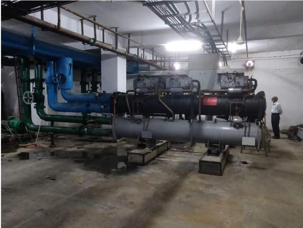
Fig. Chiller system at KGMU
