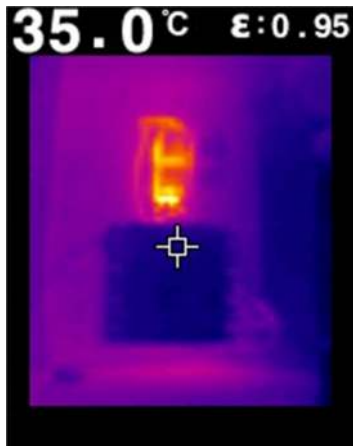
DESCRIPTION – CT FAN -1 SURFACE TEMPERATURE-35
