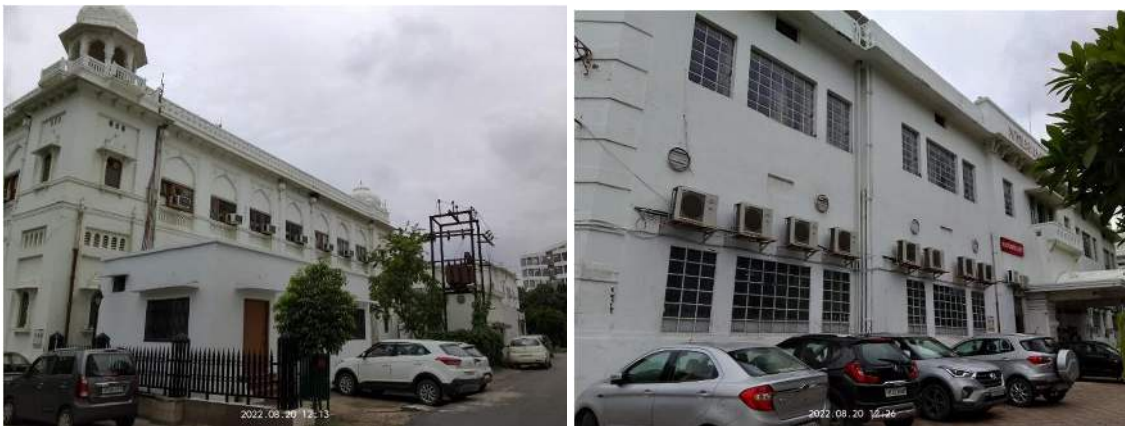
Fig. Window and Split ACs
