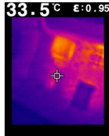
DESCRIPTION –CT FAN -3 SURFACE TEMPERATURE- 33.5
