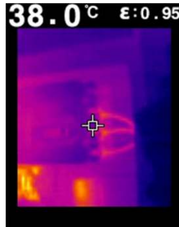
DESCRIPTION-CHILLED WATER P-2 SURFACE TEMPERATURE-38
