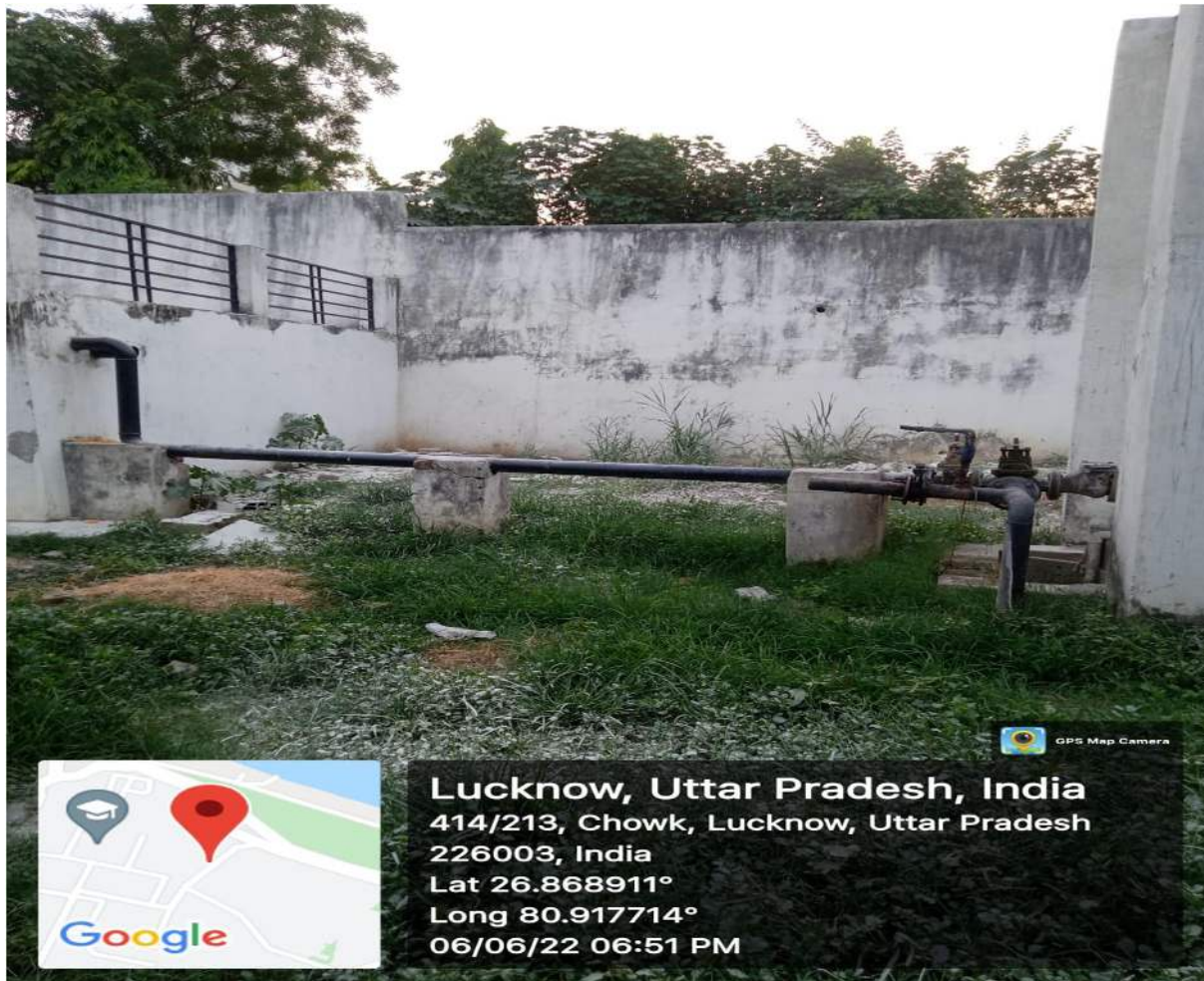
Bore well near SP Hostel for further distribution of water
