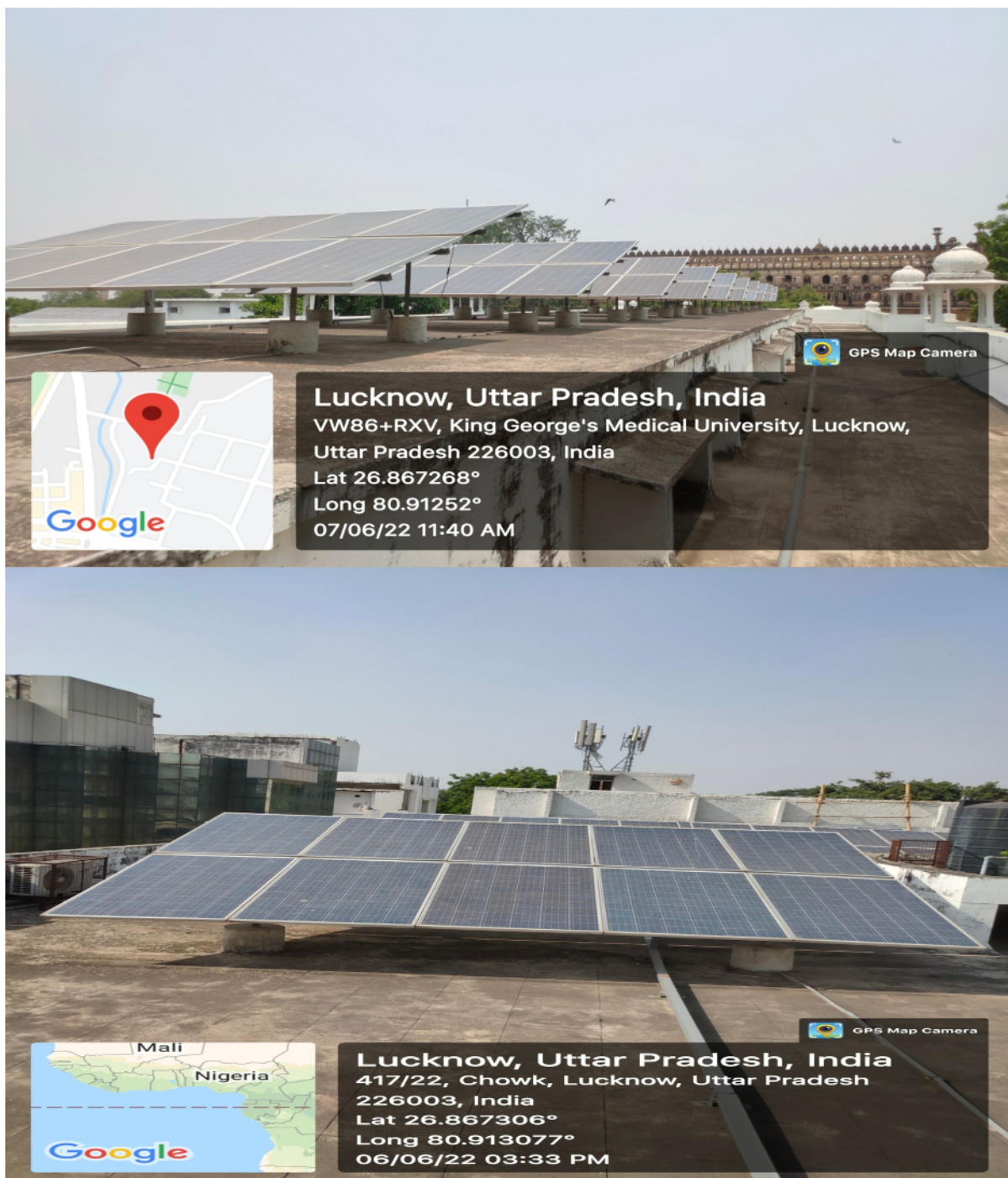
Solar Panels atop Old Administrative building and Medical Superintendent Building
