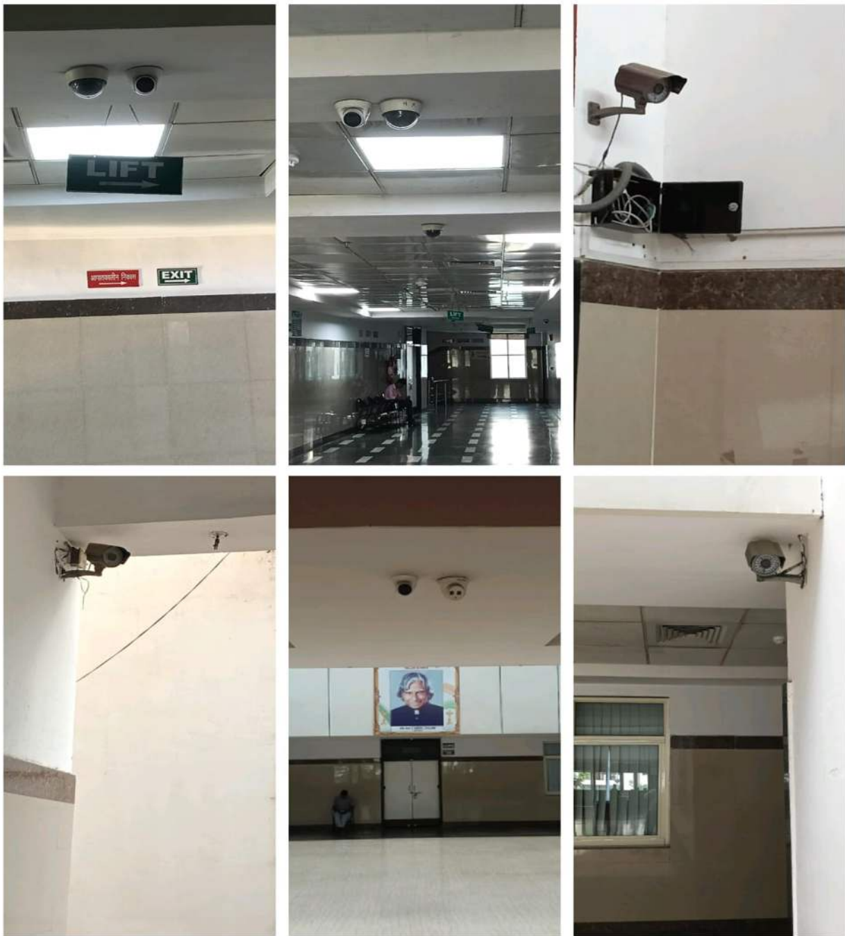
Showing the location of CCTV cameras installed at Kalam centre, Shatabdi phase 1 and 2 and Trauma center
