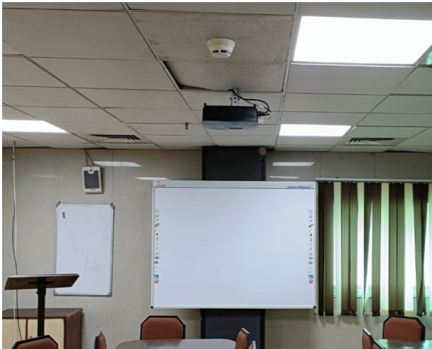
Projector in Board room
